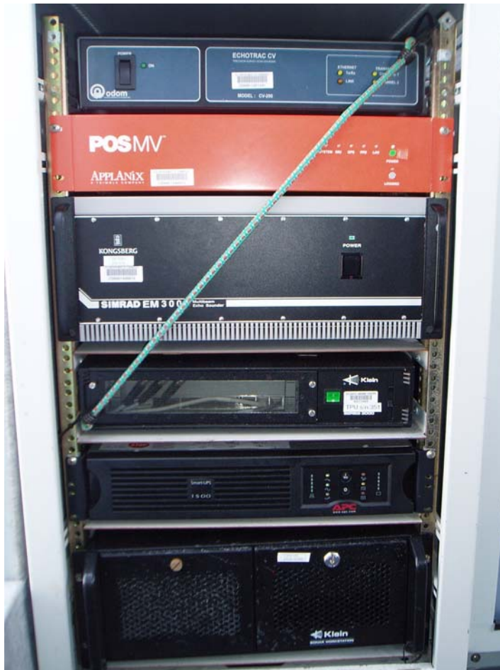
Figure 1: Rack-mounted survey hardware. From top to bottom: Odom CV Echosounder, Applanix POS/MV, Kongsberg Simrad 3000 multibeam sonar processing unit, Klein 3000 TPU, APC uninterruptible power supply, and Klein workstation.
