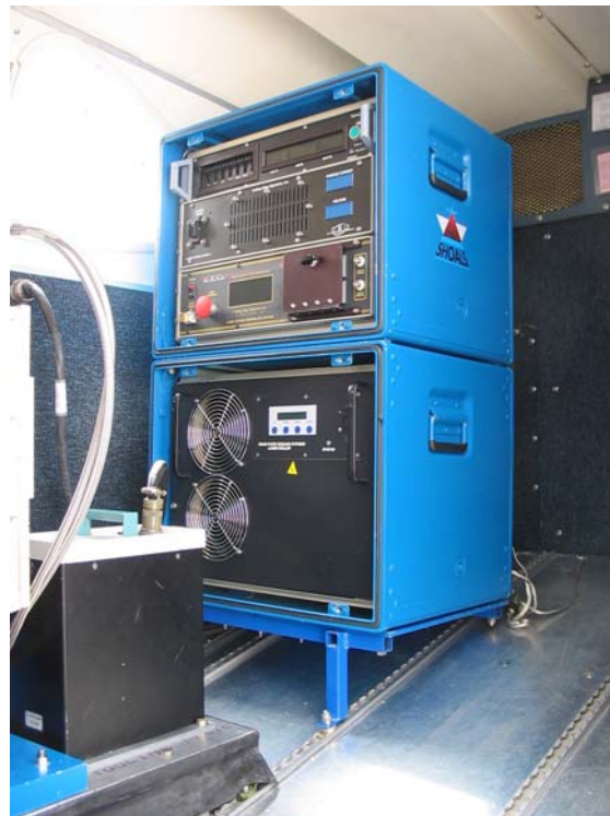
Figure B3 - System cooler and power supplies
