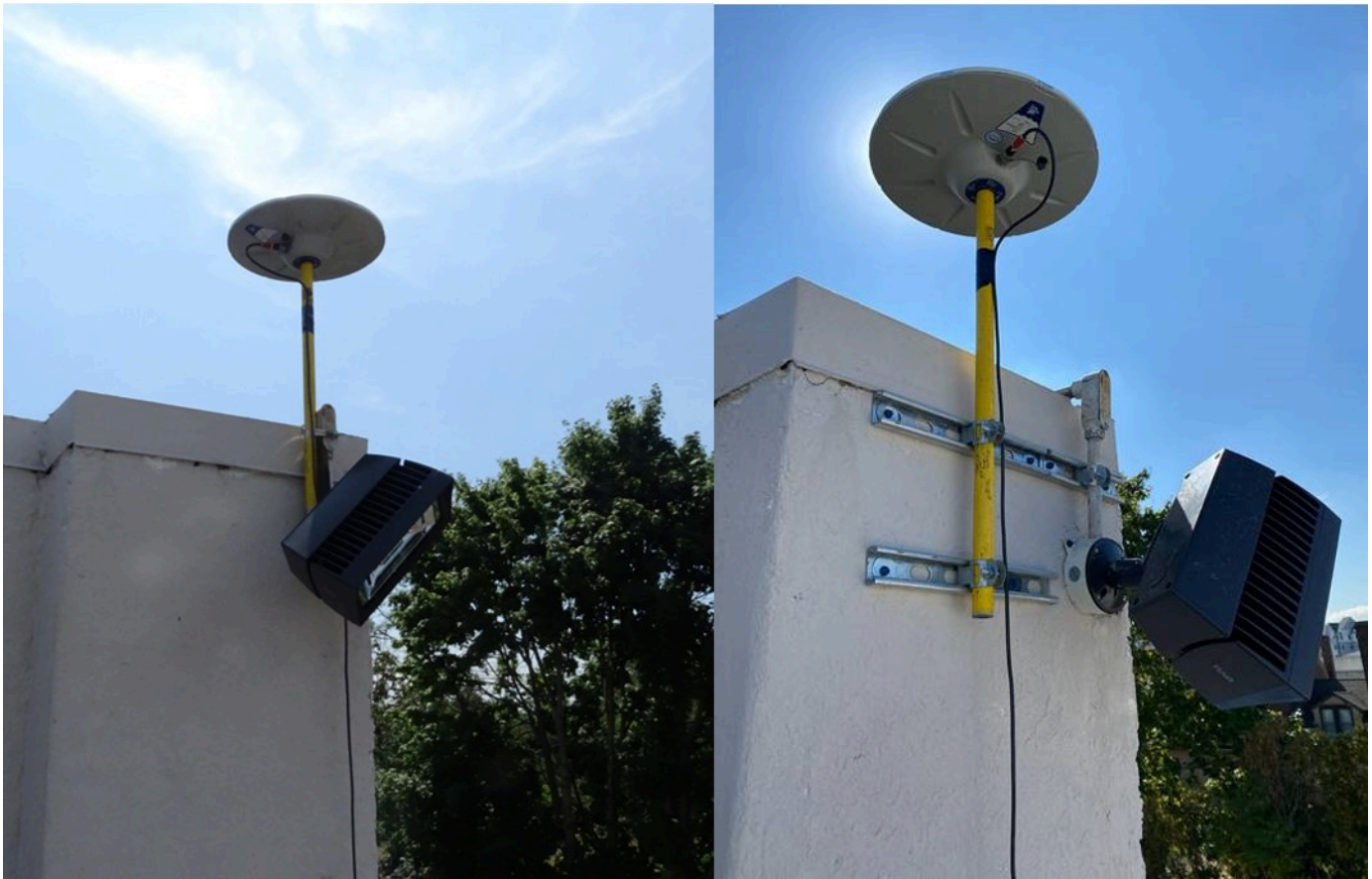
Figure 11: GNSS Base Station OSNR. Left image is original installation. Right image is the new location after 10/2/20.
