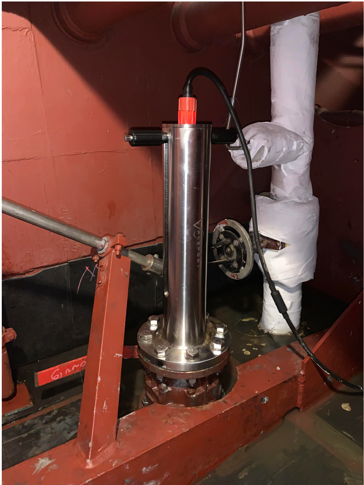
Figure 13: Valeport SVS Thruhull installation on S222
