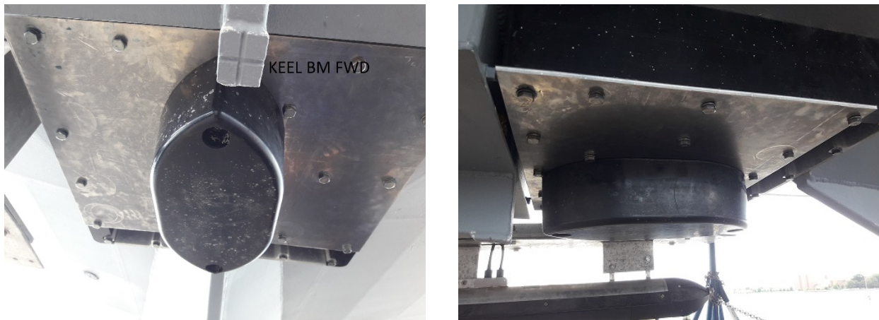
Figure 1: Installation of transducer for Odom Echotrack CV200 on the hull of TJ HSL 2903.
