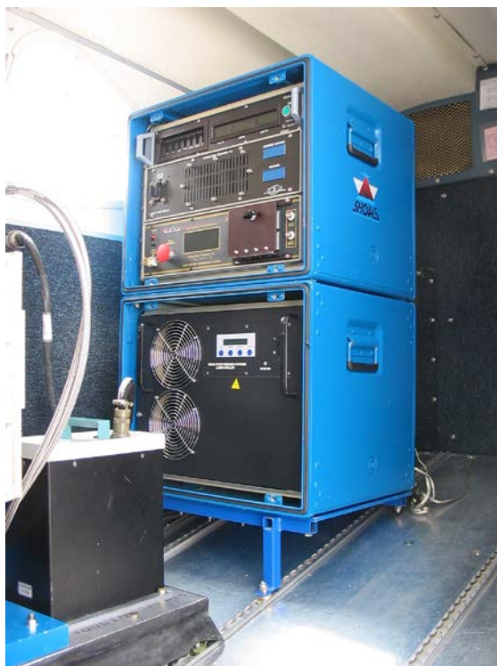
Figure B15 - System cooler and power supplies
