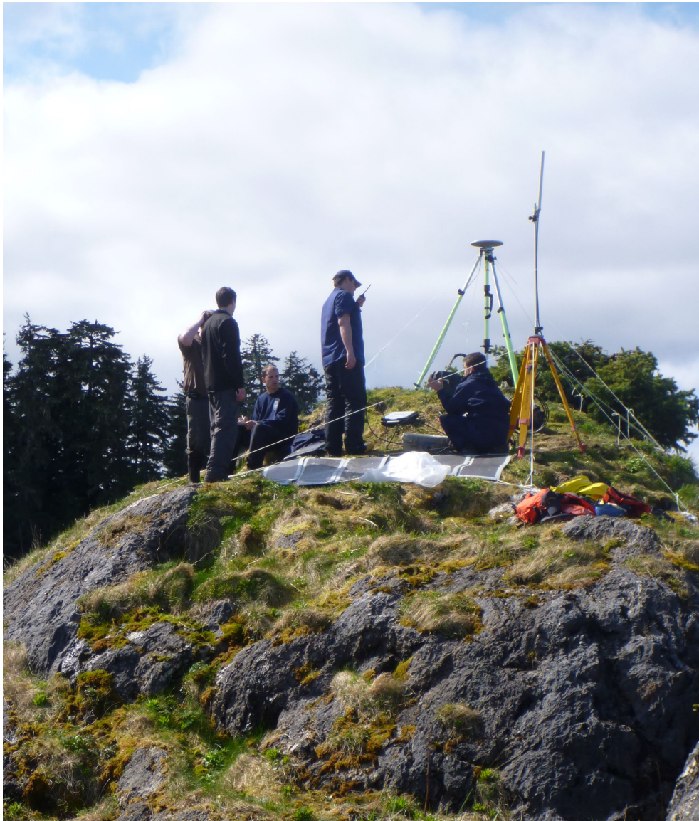
Figure 27: A Rainier base station installed in Chatham Strait, Alaska.
