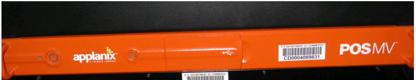
Figure 4: POS/MV computing system unit (orange) rack mounted aboard R/V BAY HYDRO II.
