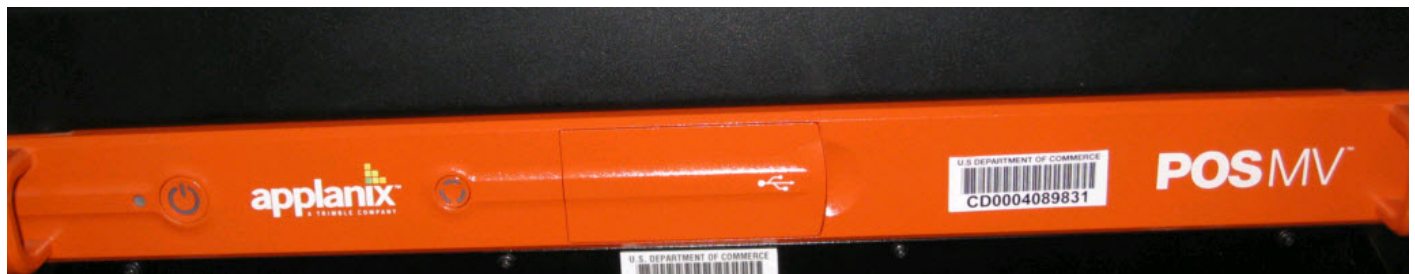
Figure 5: POS/MV computing system unit (orange) rack mounted aboard R/V BAY HYDRO II.
