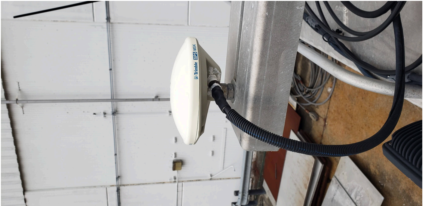
Figure 8: Temporary Secondary Antenna loaned by NRT4
