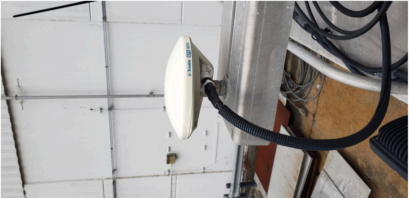
Figure 6: Temporary Secondary Antenna loaned NRB HQ
