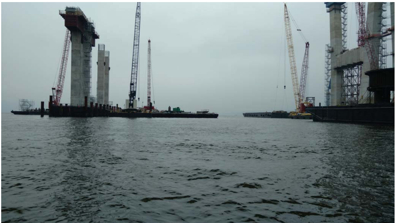
Figure 2. Barges rafted to bridge pier.
