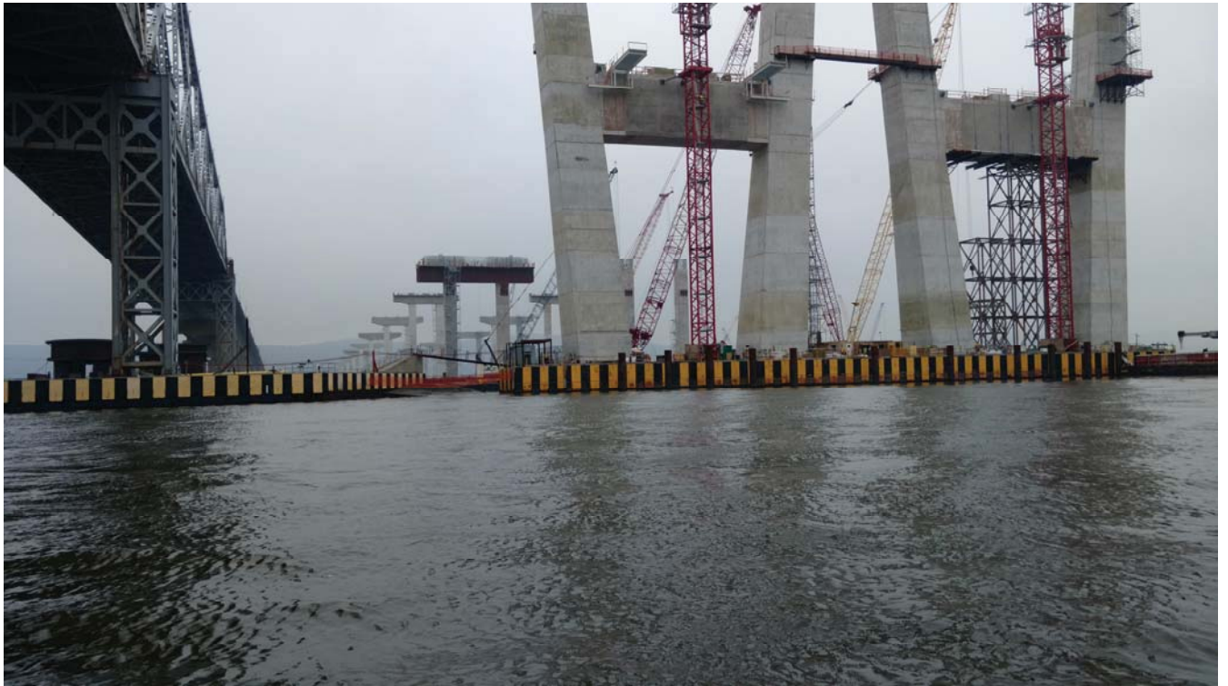
Figure 1. Overview of current Tappan Zee Bridge with new bridge piers under construction nearby.
