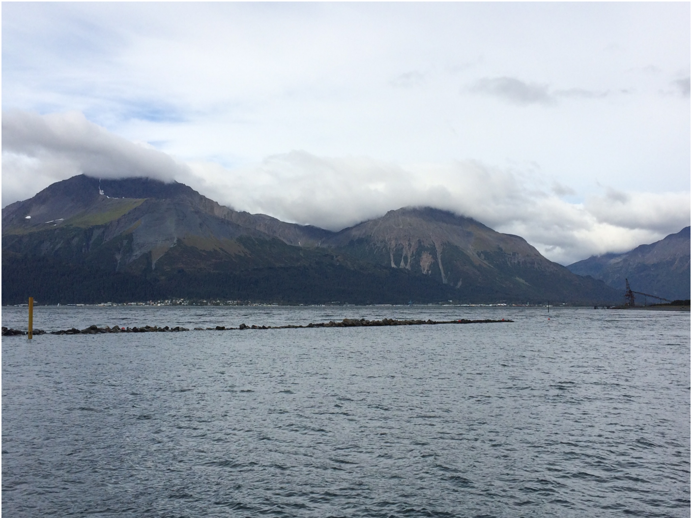
Figure 14: An images of the break water that was under construction during the time survey F00683 was ongoing.
