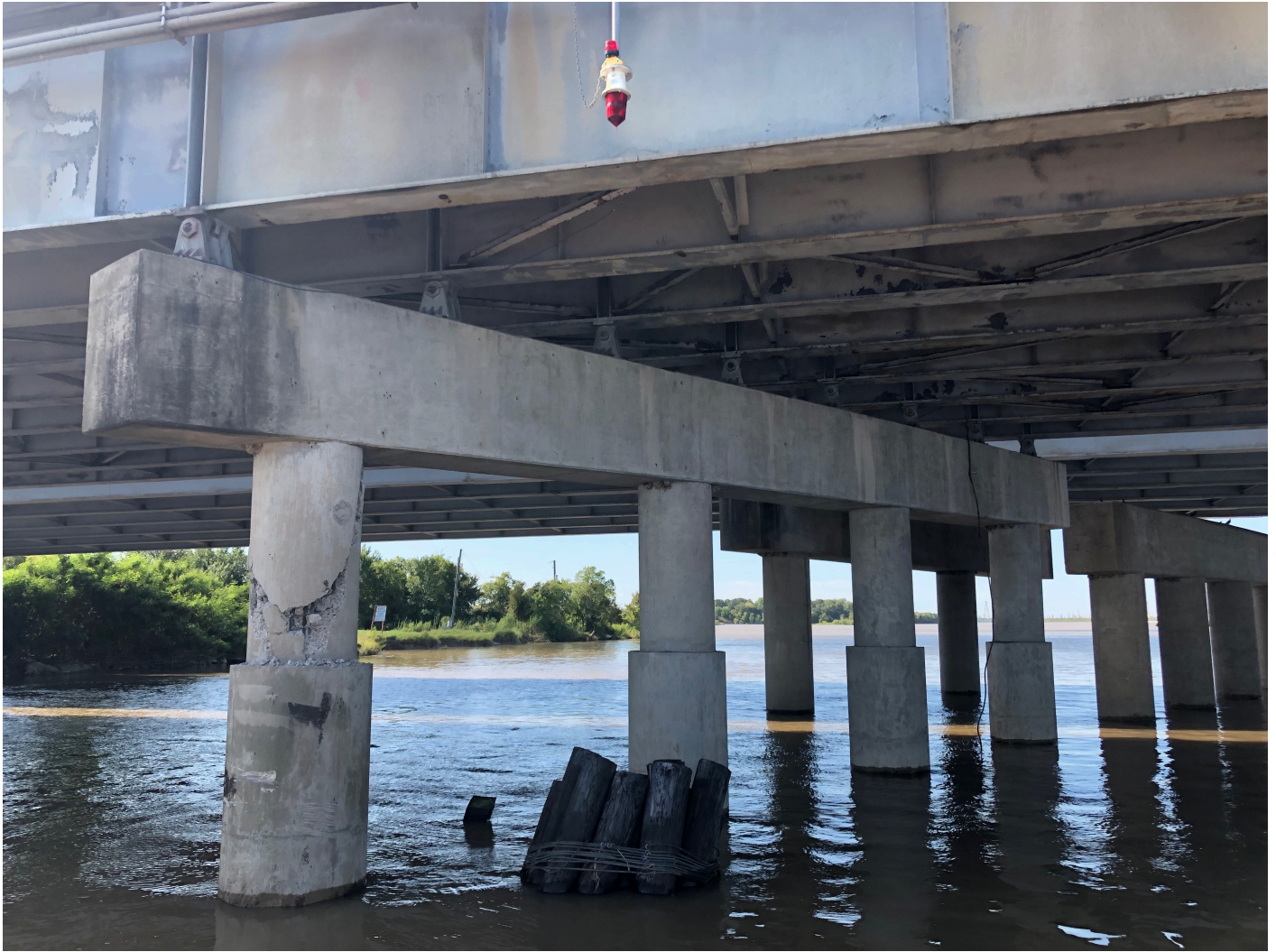
Figure 15: Cracked Bridge Pillar, Northeast side of bridge. Picture is facing South.
