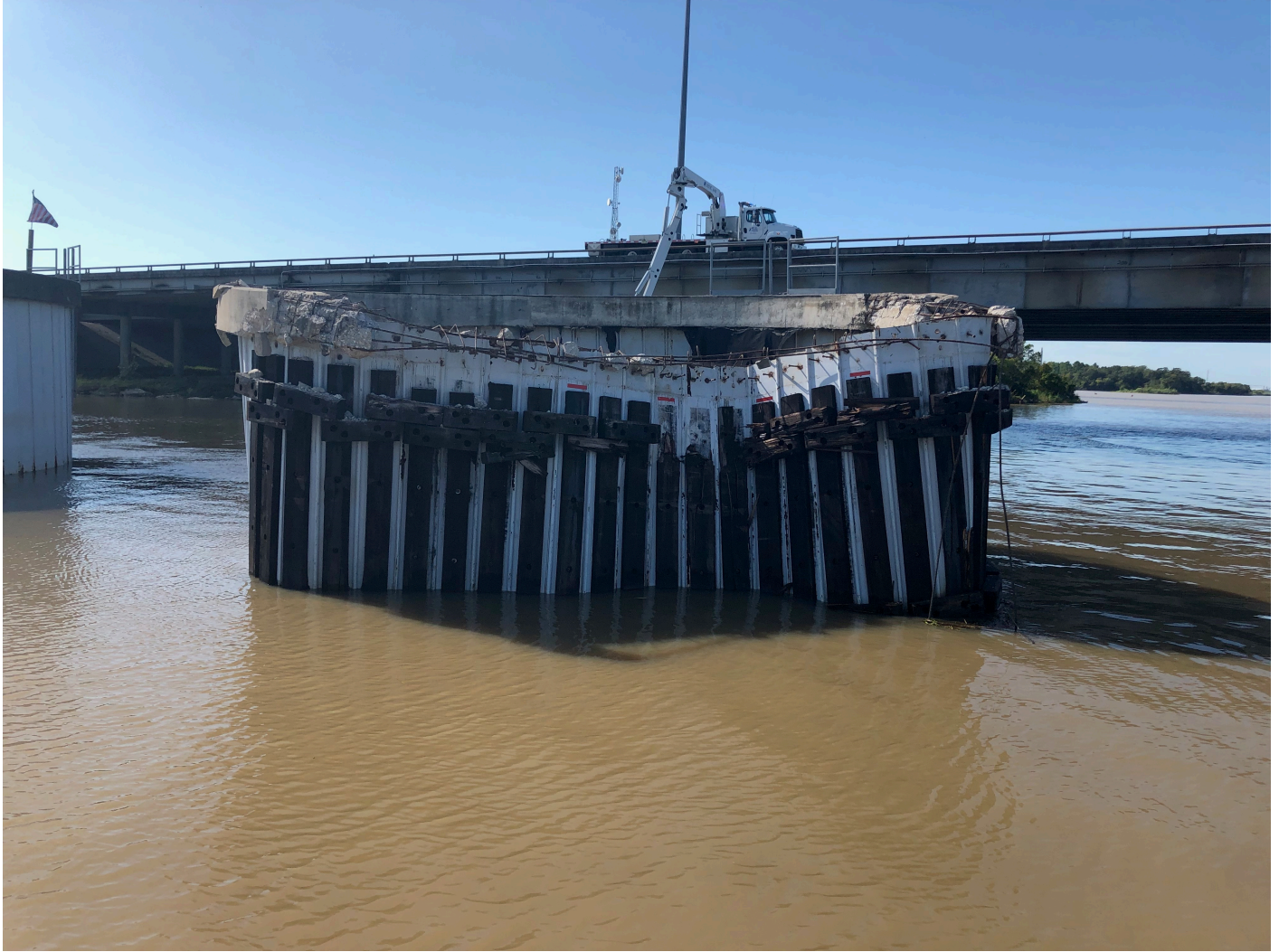
Figure 14: Damaged Dolphin, Northeast side of bridge. Picture is facing Southeast.
