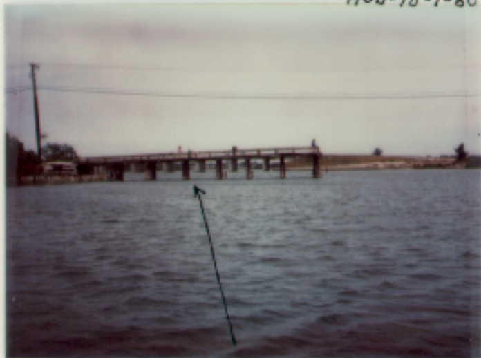
East Side of Bridge in Ruins on Audubon Rd. over Sykes Cr. Pos #81
