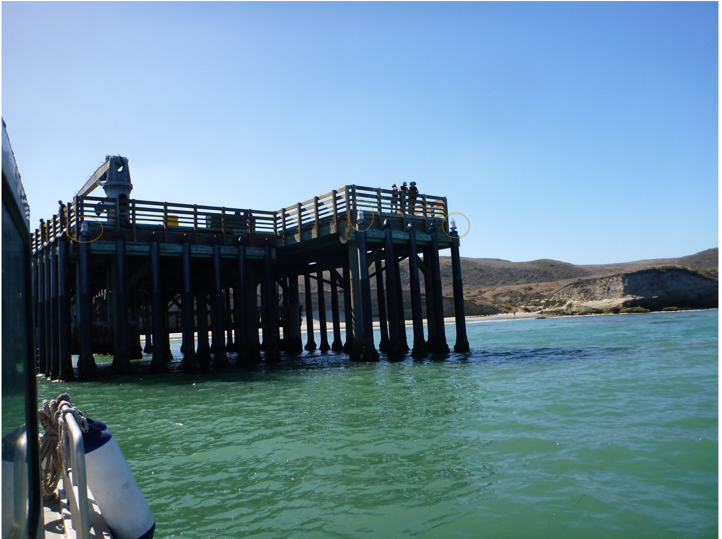
Figure 25: On the east side of Santa Rosa Island, ATONs on the end of the pier in Bechers Bay. The ATONs on this pier are privately maintained.
