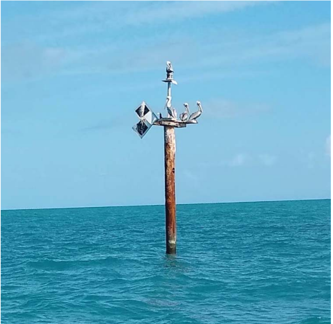
Figure 19: H13165 Visual Observation of Damaged AtoN
