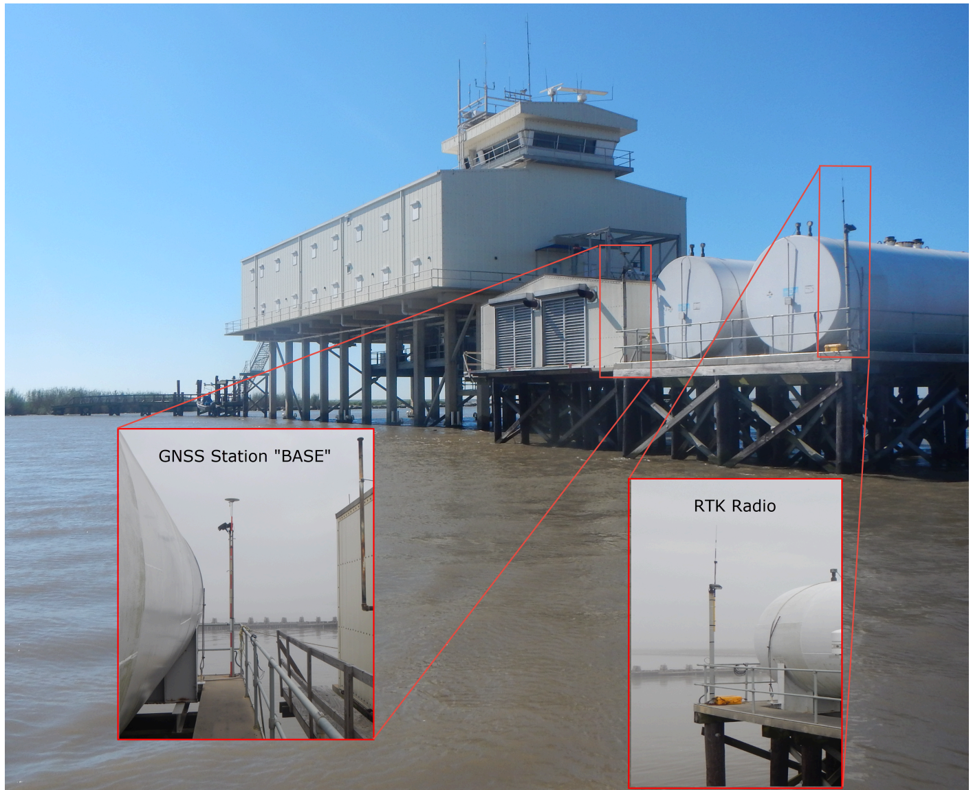
Figure 21: H13212 DEA Installed GNSS Station "BASE"
