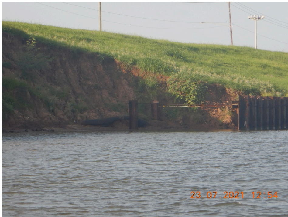
Figure 21: Photo of Eroded Coastline Along the Inner Sea Wall of Seaway Restricted Area
