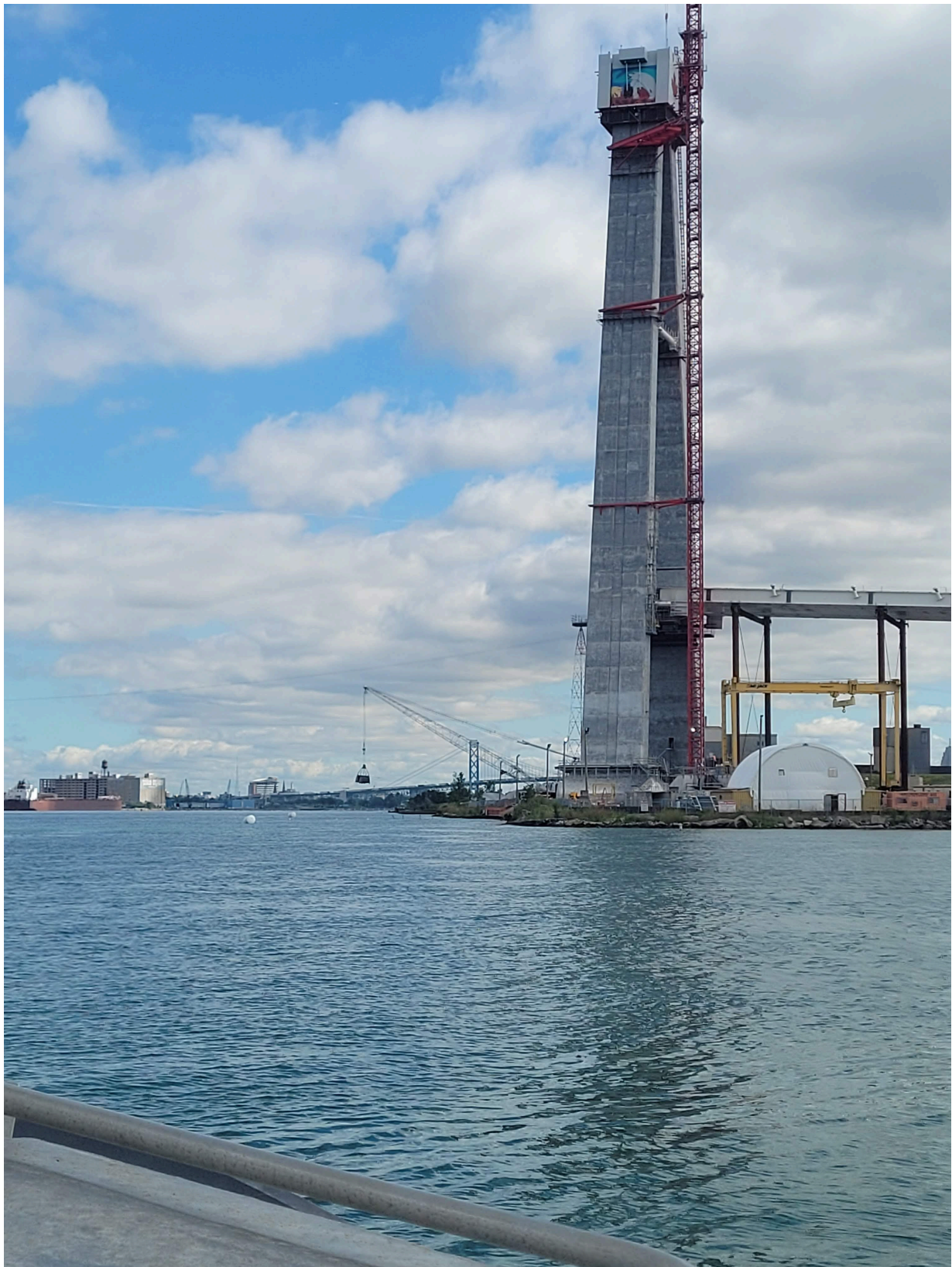
Figure 17: Active construction of the Gordie Howe International Bridge observed during survey operations in August 2022.
