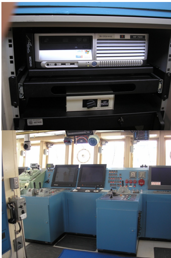
Figure 15. Bridge DP system installed on Okeanos Explorer showing different controls and the USB drive for inputting electronic files for the way point table.
