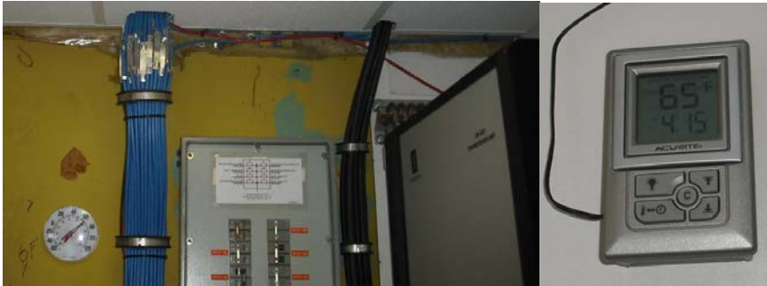
Figure 4. Photos of temperature gauges installed in the TRU closet 2009/2010 winter inport.
