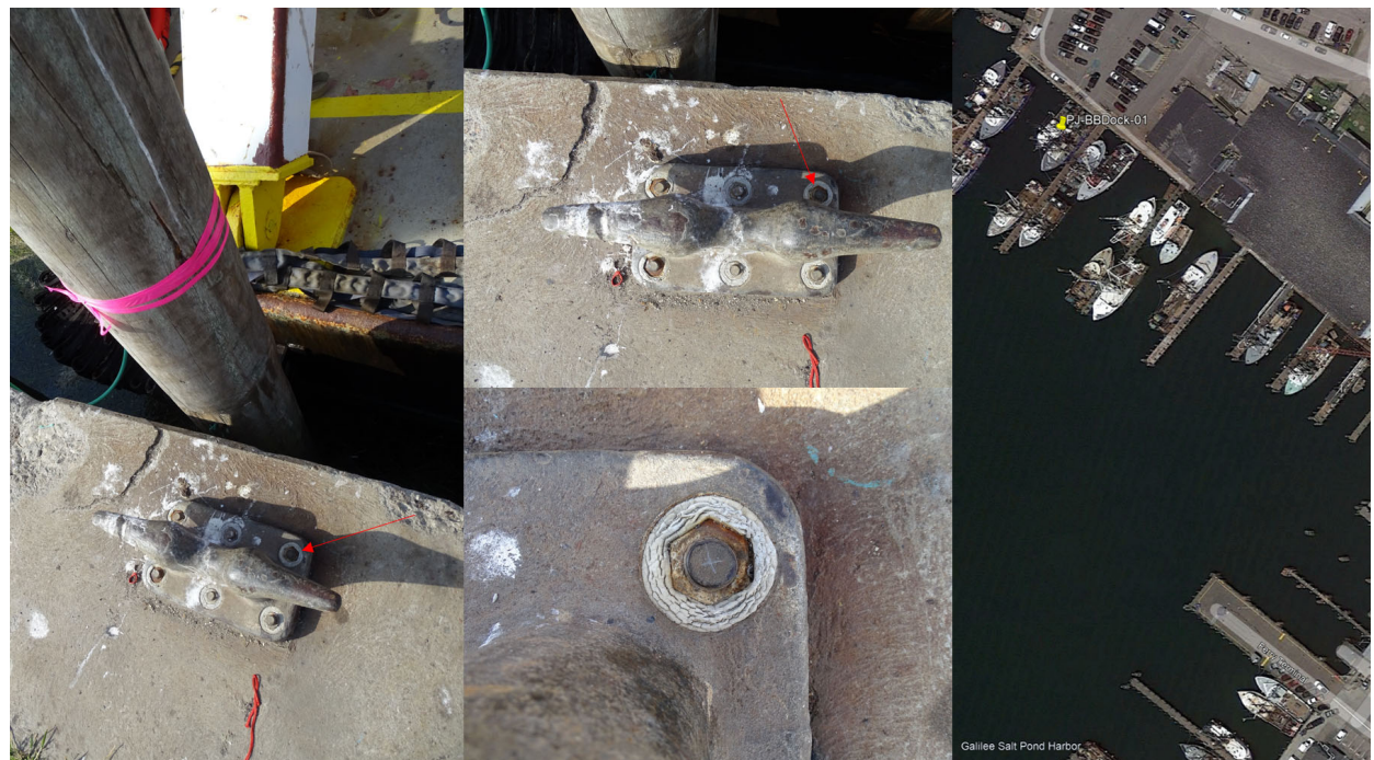
Figure 6. “PJ-BBDock-01” is the northwest bolt head on a bulkhead cleat below a pile indicated with pink survey tape located on BB Dock at Point Judith State Docks in Point Judith, RI.
